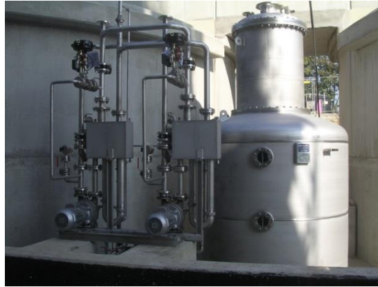
Degassing for digested sludge
