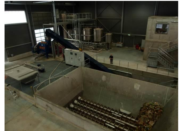
Substrate receiving and processing
